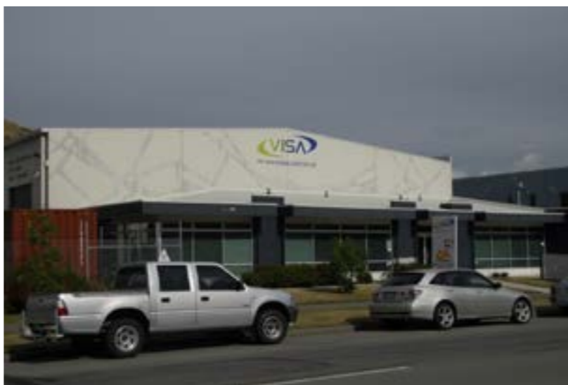
FCI VISA Christchurch - The building is still showing the scars of the earthquakes, we are hoping to have it re-painted this summer.
